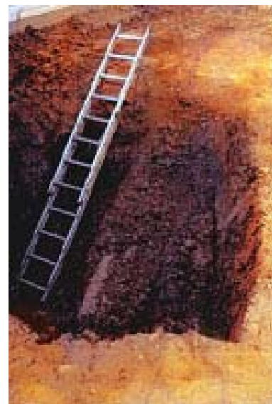
A Ladder is used as a means of egress in properly shored or sloped excavations.
